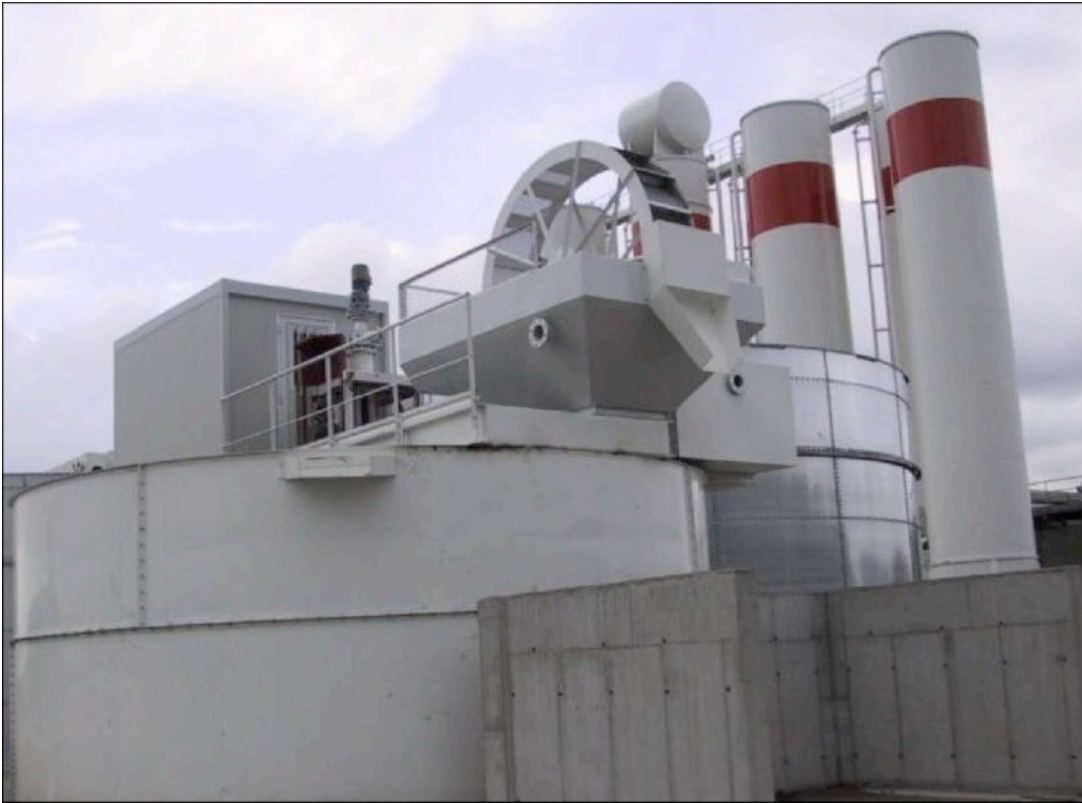
Seepage water treatment plant (Groene Hart) 200 m 3 /h
