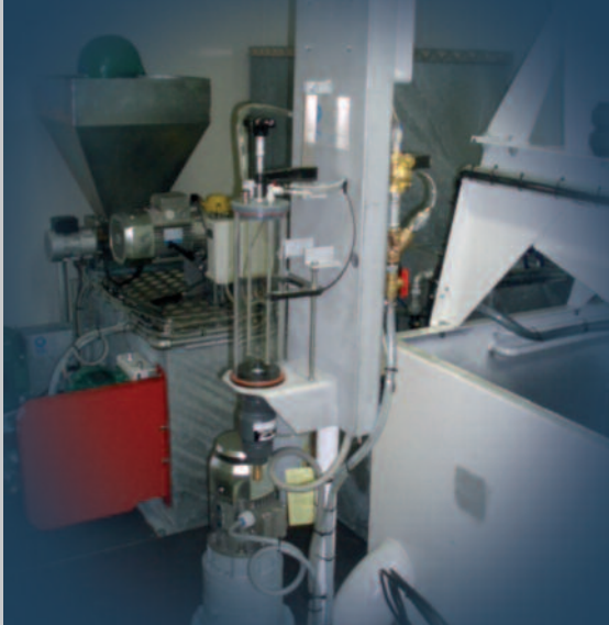
Flocculant preparation, dosing and control unit
