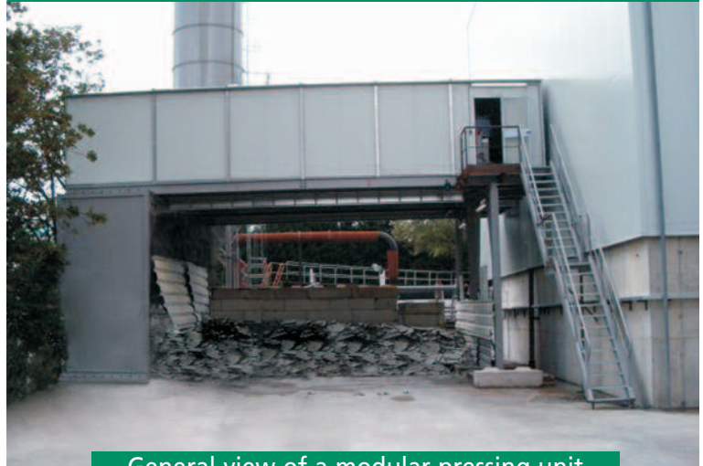
General view of a modular pressing unit
